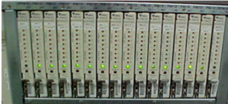
Figure 1: Server Rack with 16 cards
